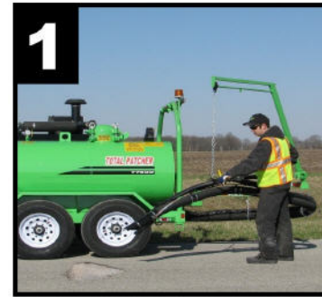
1 Clean area with on-board airstream.
